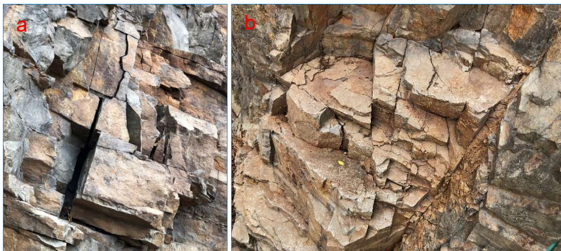
Fig. 6. a) and b) Observed loosely attached rock pieces on different locations on rock slope (Project 1)
