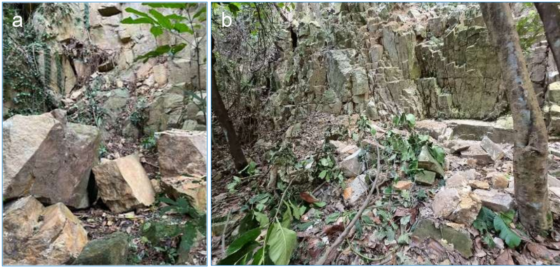
Fig. 14. a) Observed recent rock fall at Project 2 and b) Observed recent rock fall at Project 2
