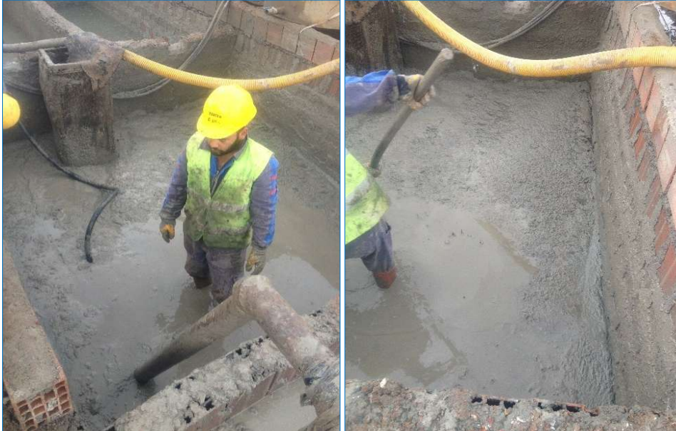
Fig. 6. Views of the flocculation in the mud pit and discharging the flocculated mud from the pits
