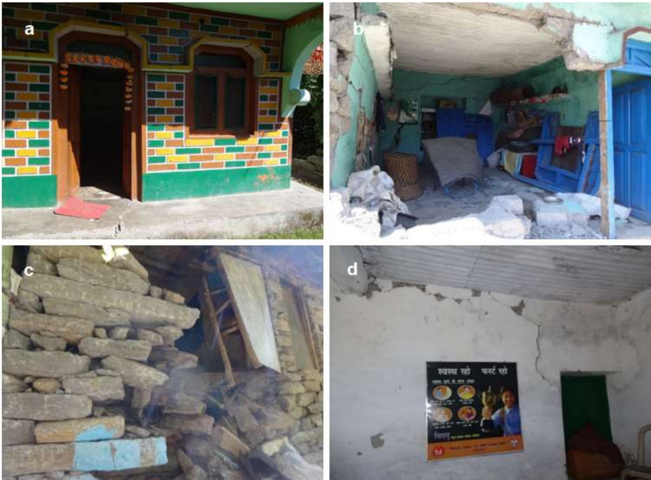
Fig. 17. Cracks in houses of Khela Village due to creep movement; (a) cracks in house at Ala Tok, (b) severely damaged house at Kolpani Tok, (c) damaged right-side wall of traditional house at Chetkala Tok and (d) cracks on roof column and wall of primary school at Chetkala Tok
