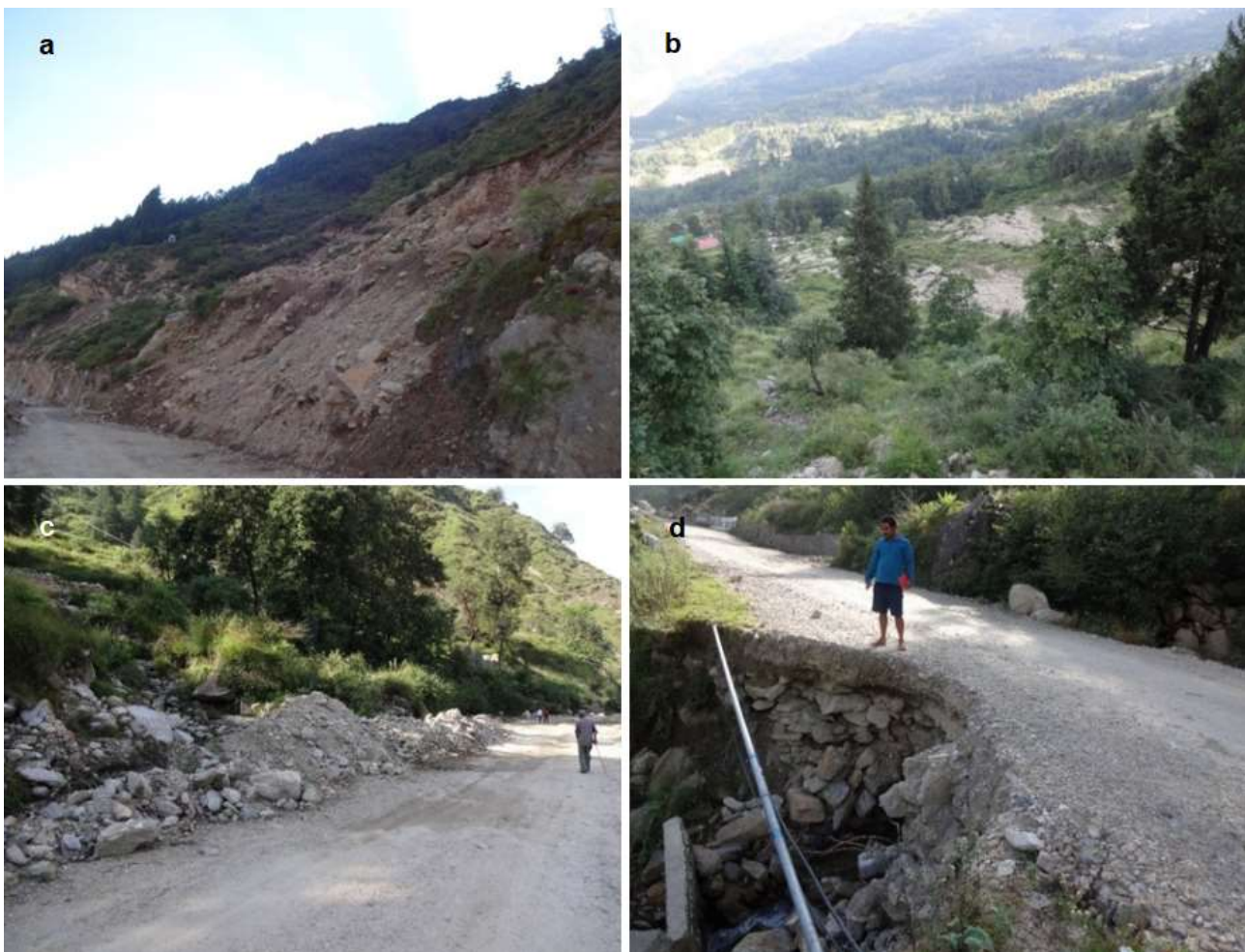
Fig. 5. Heavy rains triggered debris flows and related damages in Balta Tok; (a) undercutting of hill slope for road widening; (b) debris flows from uphill road overrun agricultural fields and houses; (c) severely damaged culvert due to excessive water saturated debris discharge by local stream; (d) unlined and chocked hill side drain on road due to debris flows
