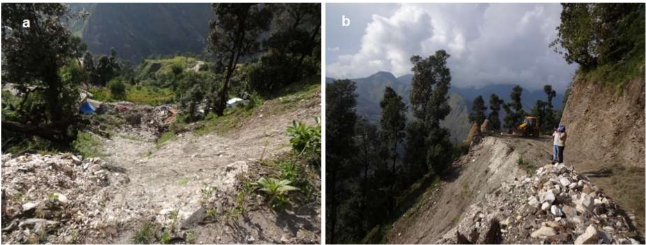
Fig. 12. Slope failure at Gaila Malla Tok in Pattharkot Village; (a) failure slope above destroyed house (b) damaged portion of under construction road
