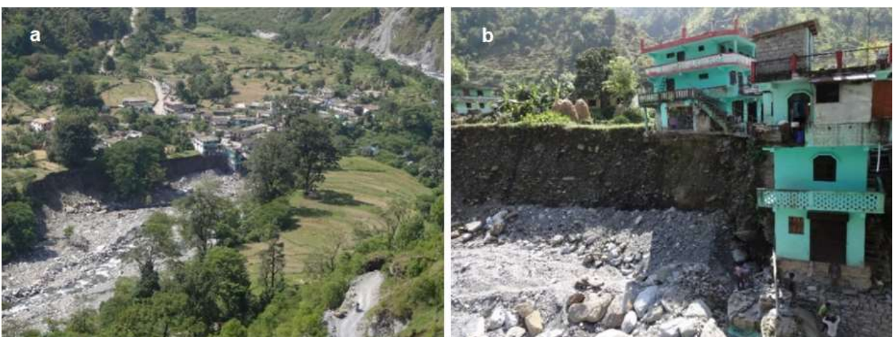
Fig. 14. View of eroded terrace with houses in vulnerable state on the left bank of Barar Gad; (a) panoramic view and (b) close view
