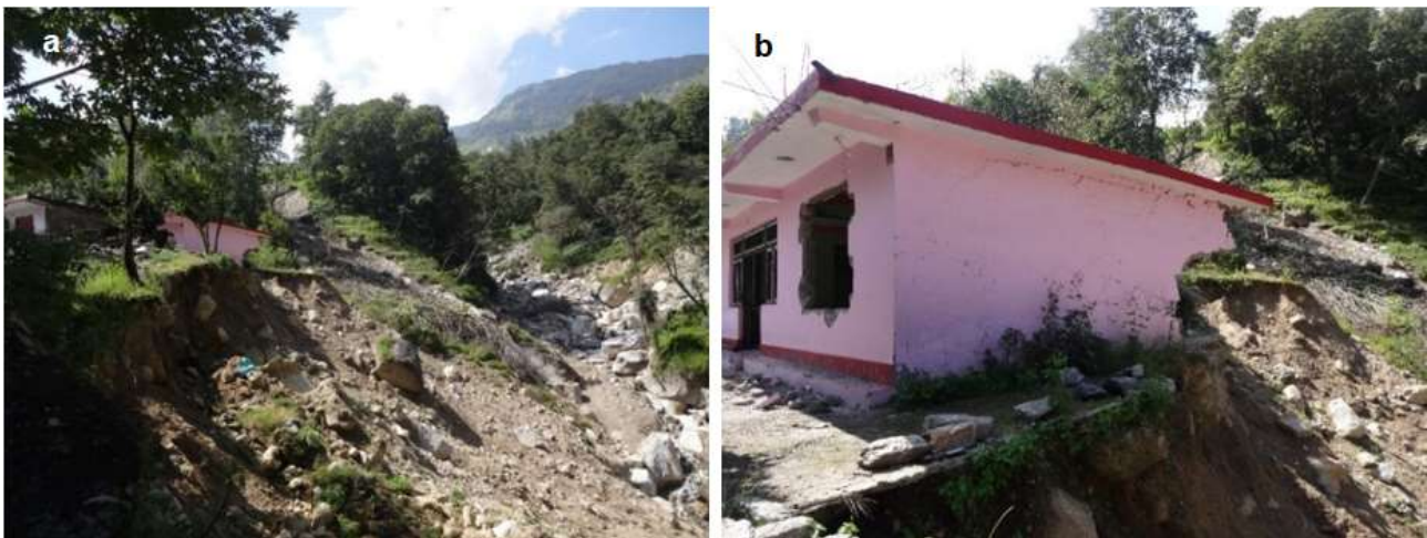
Fig. 8. Severally damaged a house due to toe erosion by Dhapwa Gad; (a) on the edge of failure terrace and (b) close view of the same house
