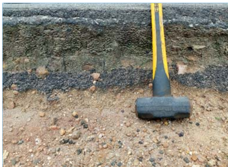
Fig. 10. Section of the exposed highway structure at Ogbese, where existing design thickness was measured to be 315 mm
