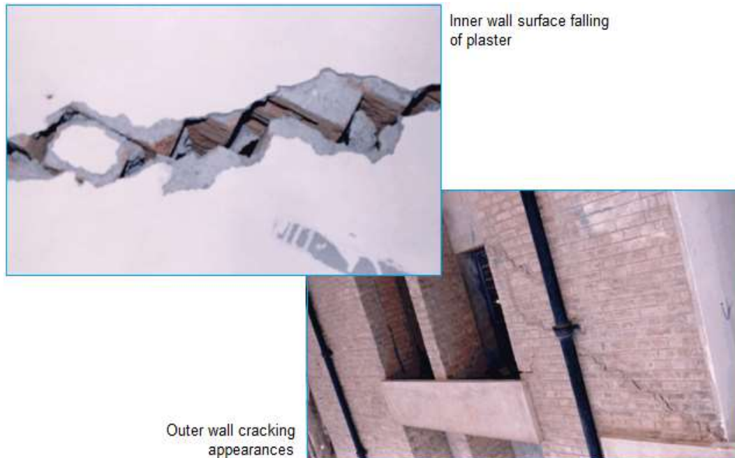
Fig. 6. Fissure and cracking on the wall after earthquake impact
